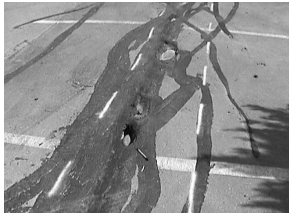
Photo 4 – Close-up of Pavement Cracking with Sinkhole
