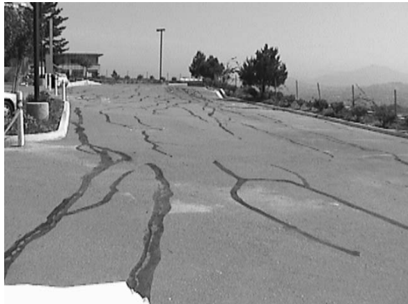
Photo 3 – Extensive Pavement Cracking Behind Wall
