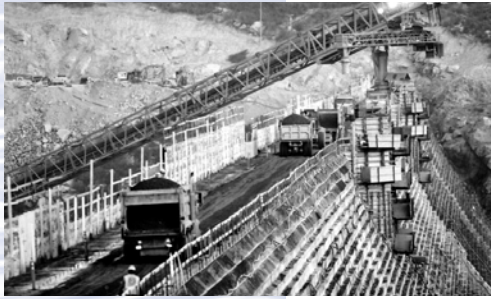
Roller-compacted concrete will be used to raise the dam, which was also used to construct the Olivenhain Dam in 2003.
