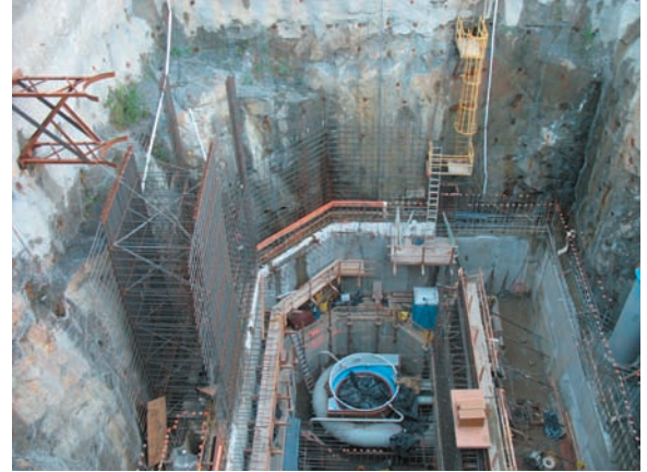
Impellar housing. Photograph courtesy of Gregory Farrand.
